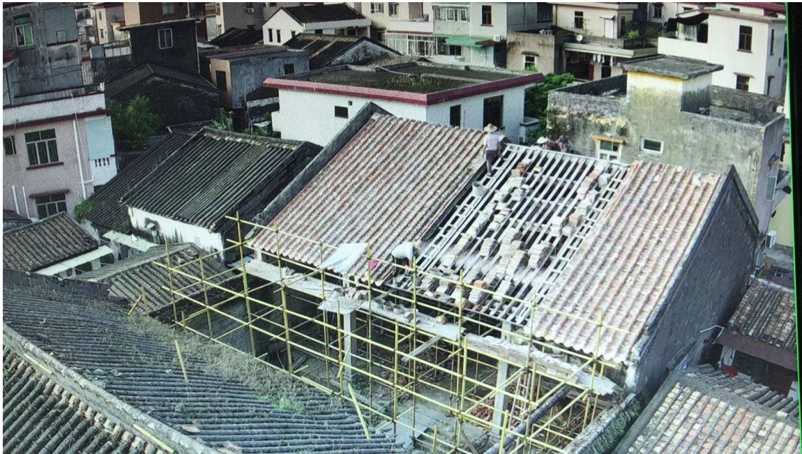
Old roof left of the scaffolding. Right: new roof installation in progress.
